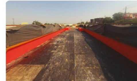
The polyurea needed to be protected before rocks and rail were installed on top. The crew used 1/2-in (1 cm) asphaltic board on the vertical and horizontal surfaces. Photo courtesy of Mobile Enterprises, Inc.
