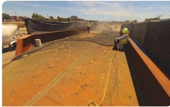
A crew from Mobile Enterprises Inc. was surprised to see weathered steel on two new spans for a rail overpass project in Plano, Texas. Sandblasting to prepare took much longer than expected. Photo courtesy of Mobile Enterprises, Inc.
