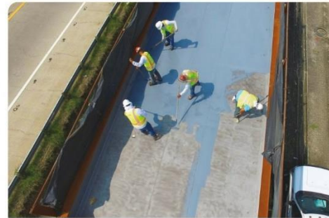
To hold the blast, the crew immediately applied a thin layer of Bridge Preservation's Multi-Use Primer FAST using squeegees and rollers. Photo courtesy of Mobile Enterprises, Inc.
