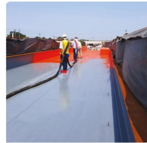
The Bridge Deck Membrane, protective polyurea was applied to an average of 120 mils (3,048 µm). Photo courtesy of Mobile Enterprises, Inc.
